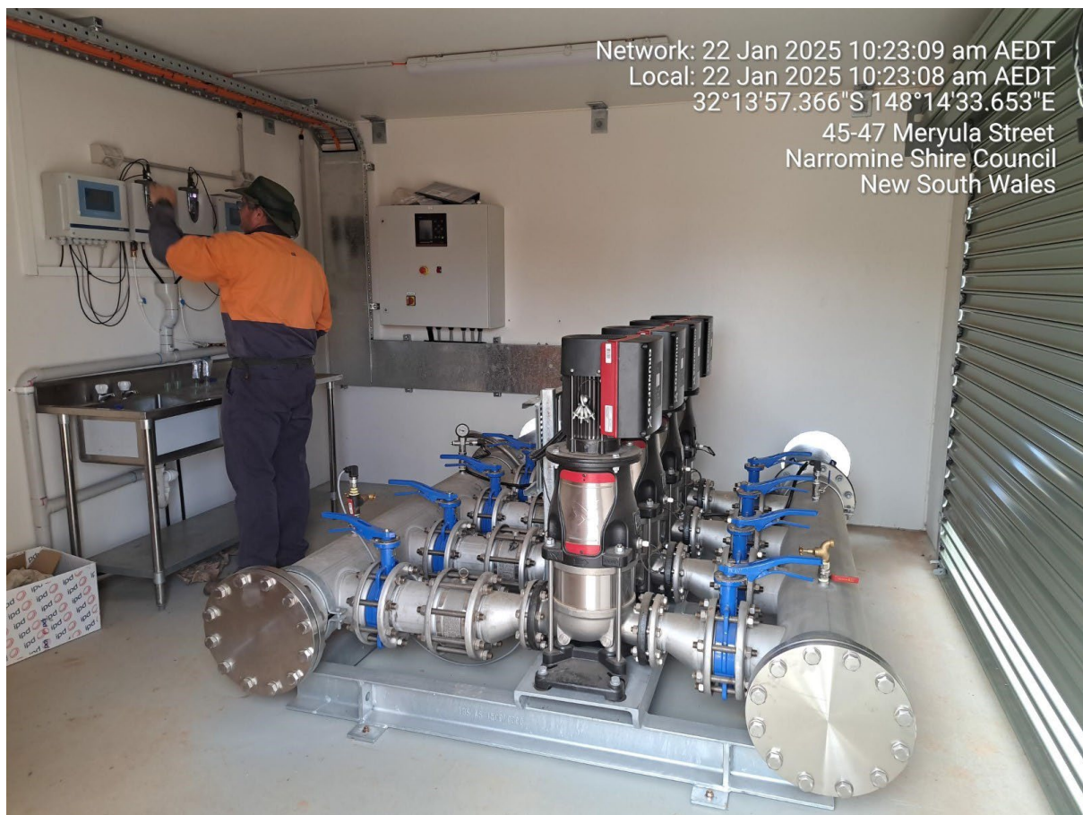
Figure 1: The booster pump station at Nymagee Street is now operational
